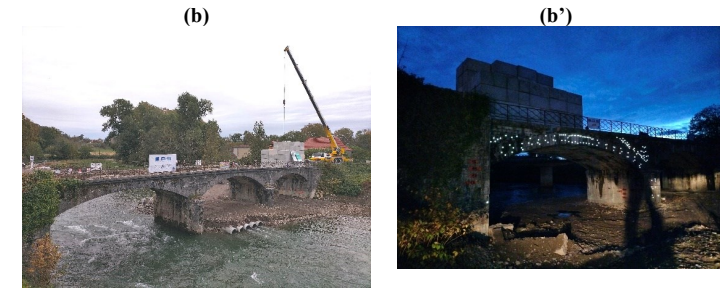
Figure 1: Photos of (a) the retaining wall and motion capture system and (a') the \varnothing 19 mm markers, (b) the loading of the bridge and (b') the reflective markers by night
